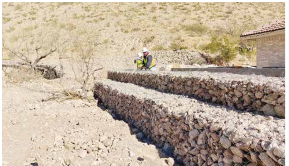
Contractors building gabions (wire cages with rocks) at the Memphis Dam in Central El Paso.
